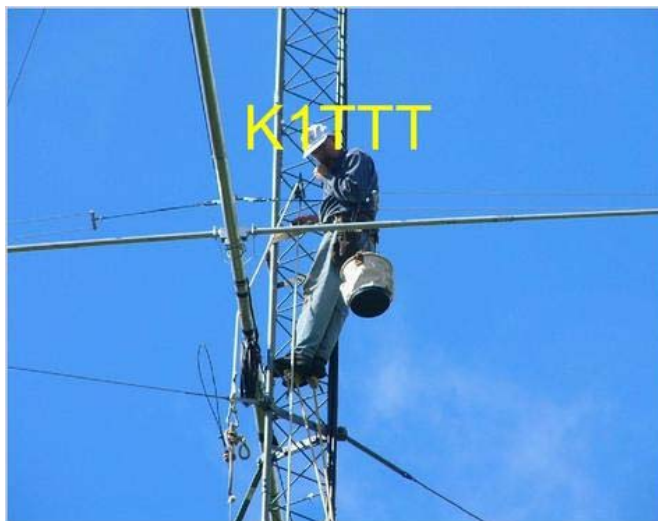
Antenna work being performed on one of the many towers at the K1TTT station.
